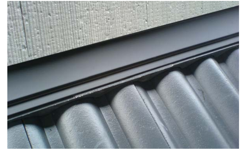
h-h' 〔Wall boundary (Horizontal direction)〕 壁際 (水平)
